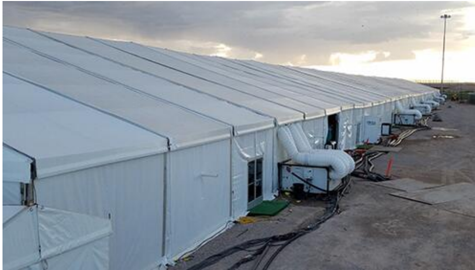
The temporary facility built to hold 2,500 single adults in Tornillo, Texas, is scheduled to open Friday.
